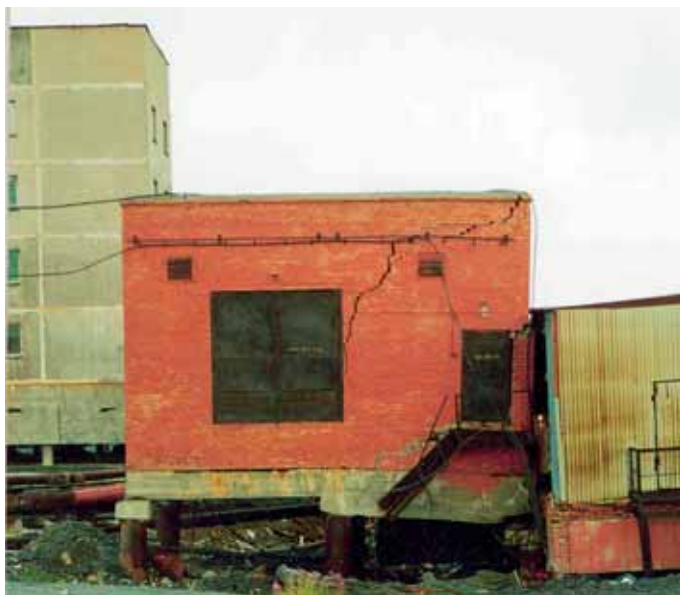
Fig. 2. Thawing of an ice-rich permafrost in the area of installation of underground utility line and resulting deformation of structure in the residential area of Oganer near Norilsk. July 2003
