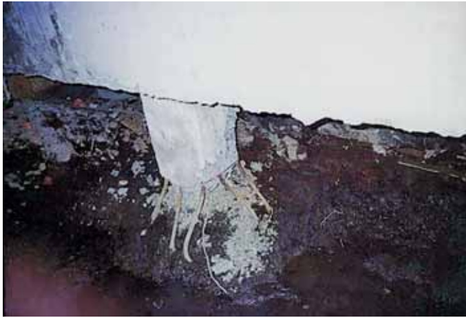
Fig. 4. Bands of "frost destruction" of reinforced concrete piles within the active-layer, Norilsk
