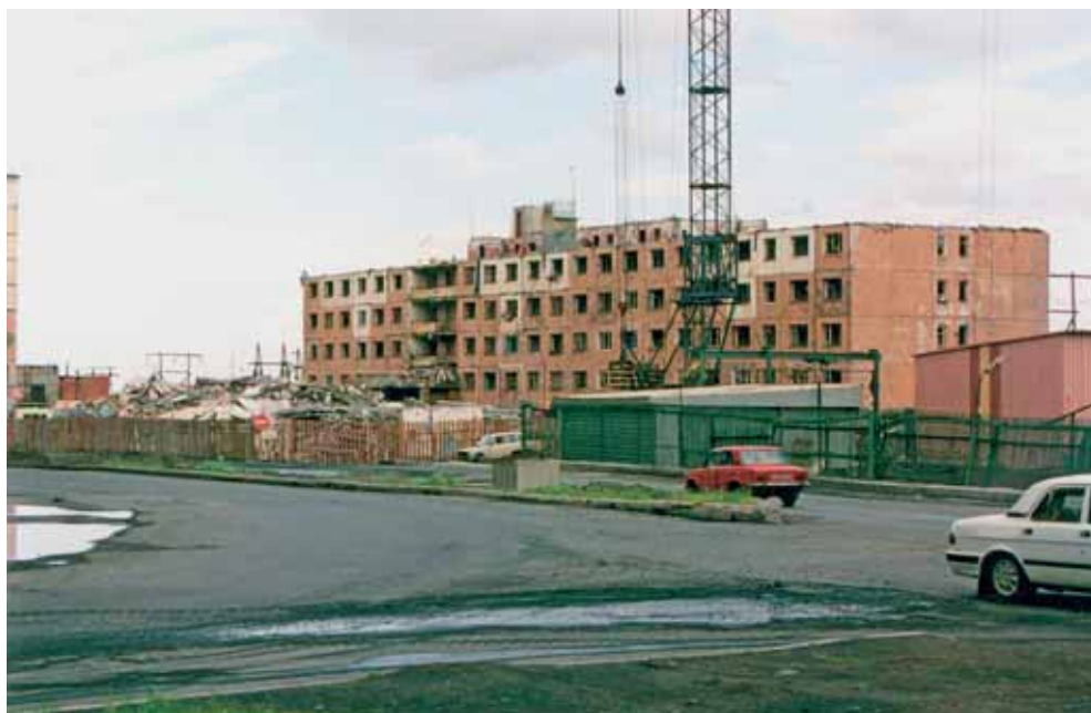
Fig. 3. Demolition of a nine-story residential building on Laureates St. in Norilsk after 21 years of operation, July 2001
